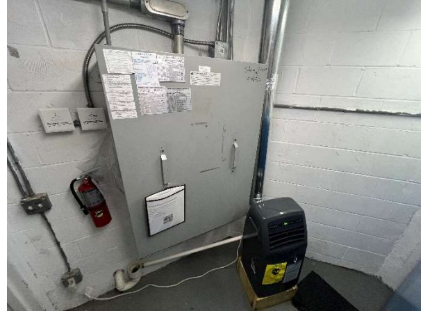
Hydraulic elevator controls
