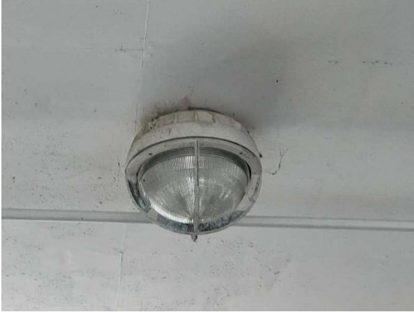
Garage light fixture
