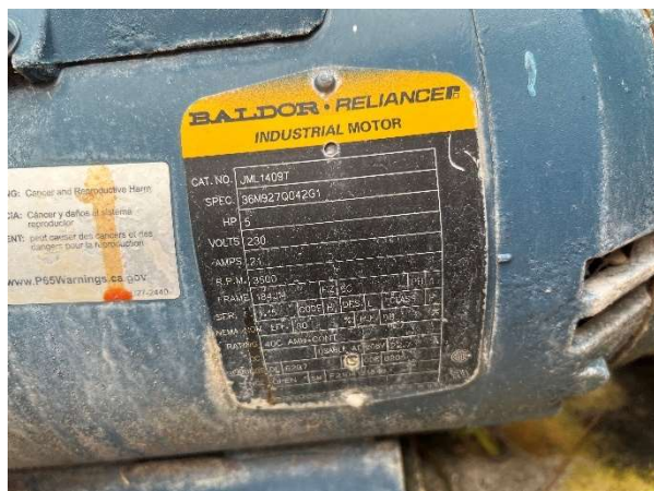
Irrigation pump placard
