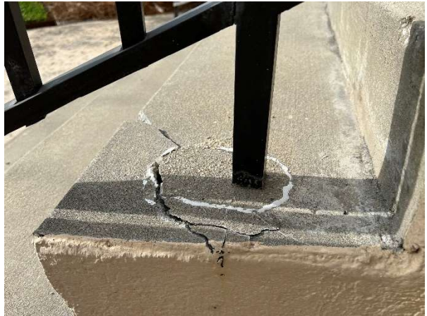
Railing and concrete damage at rear steps
