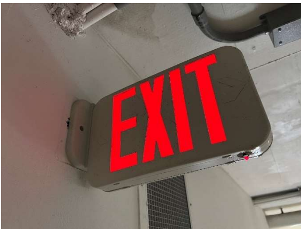
Emergency exit light
