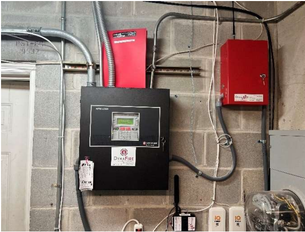
Life safety control panel area
