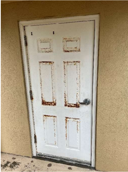
Rust evident at exterior doors
