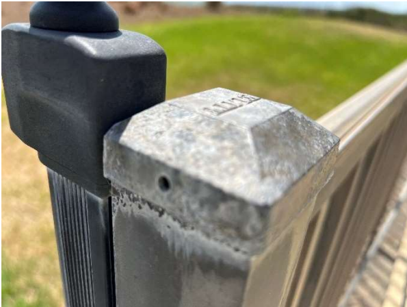
Post cap deterioration
