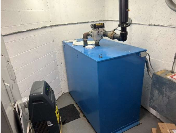
Hydraulic elevator equipment
