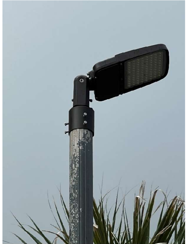
Recently replaced fixture with pole finish deterioration
