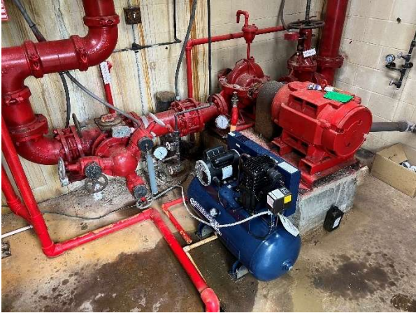
Fire suppression pumps and compressor
