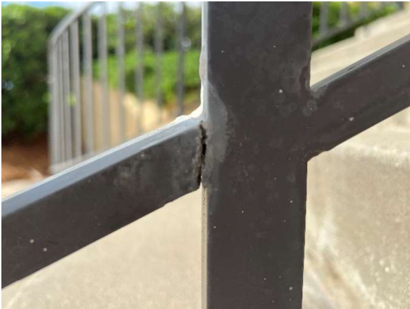
Railing damage at rear steps
