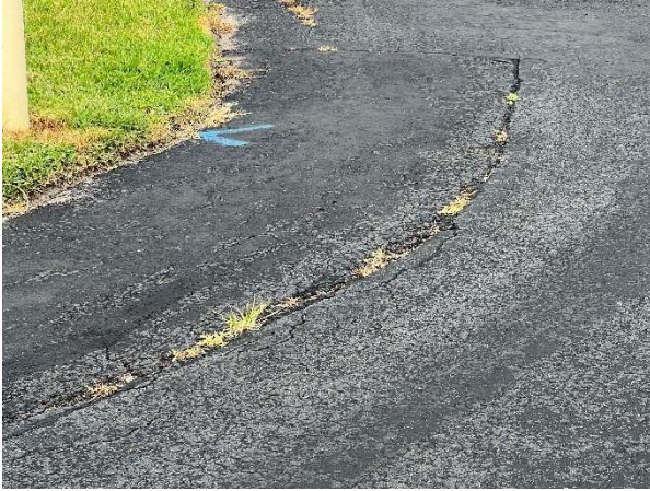
Cracks with vegetative growth evident
