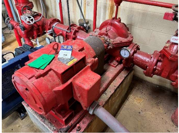
60-HP fire suppression pump
