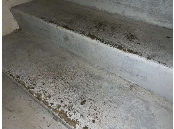
Tread coating deterioration
