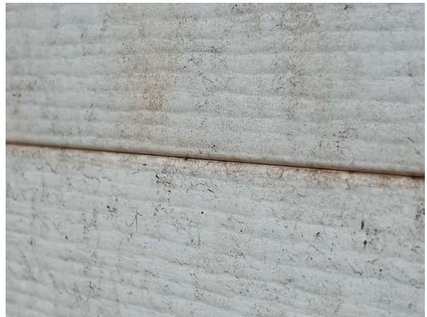
Faded and deteriorated finishes at garage door
