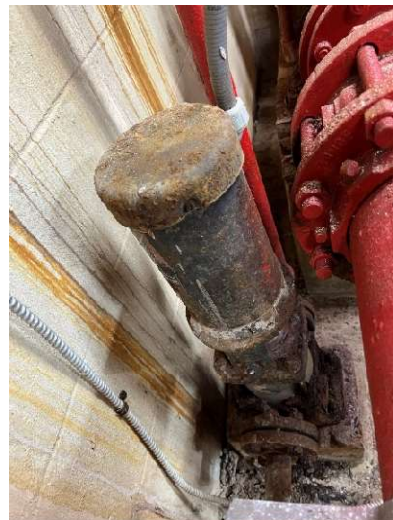
Corroded jockey pump
