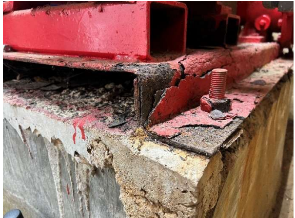
Corroded frame and mount
