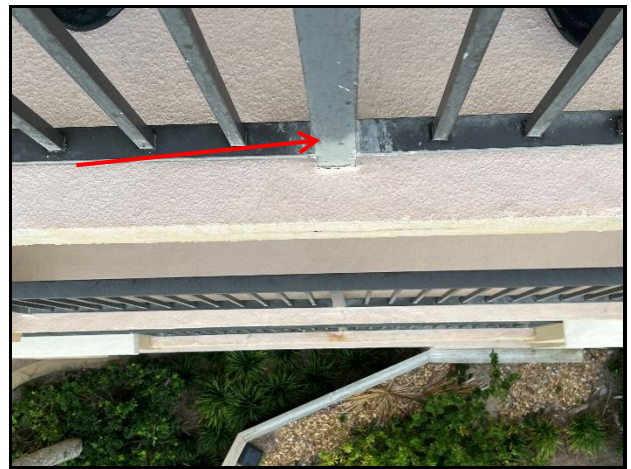
Photograph 8. Rail paint fading and deteriorating.
