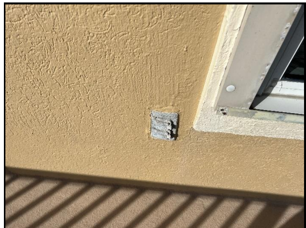
Photograph 20. Corroded outlet cover.
