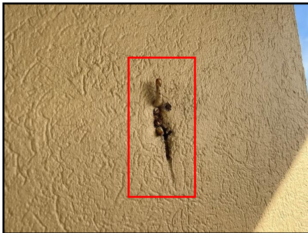
Photograph 15. EIFS impact damage.
