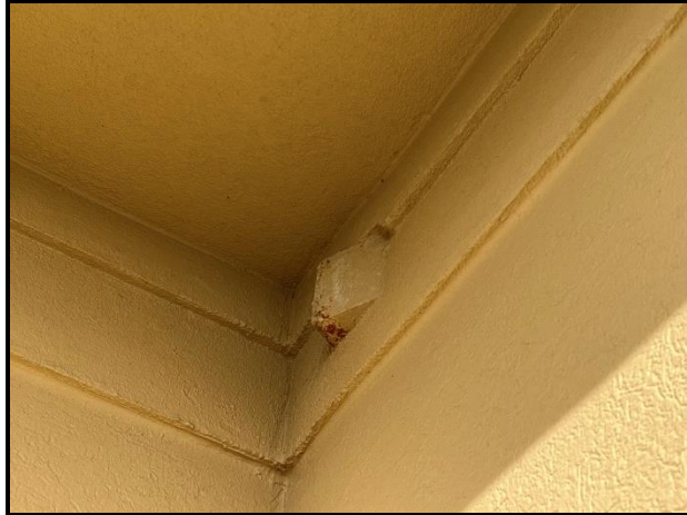
Photograph 17. Vent cover corroding.
