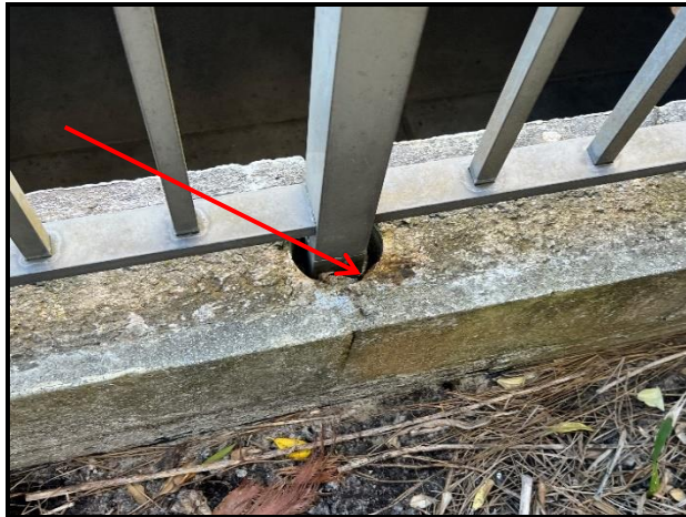
Photograph 29. No waterproofing installed on CMU wall, post pockets failed.
