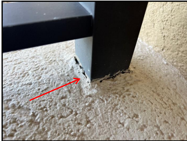
Photograph 11. Failed rail sealant.
