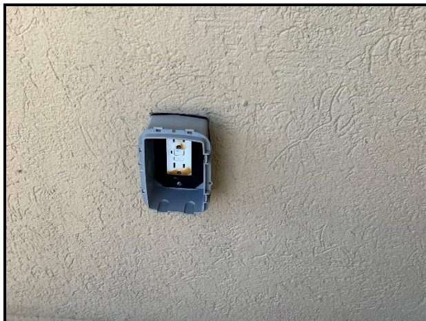
Photograph 19. Missing outlet cover.
