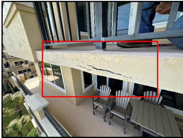
Photograph 1. Balcony edge spall, note location of core mount directly above the spall.
