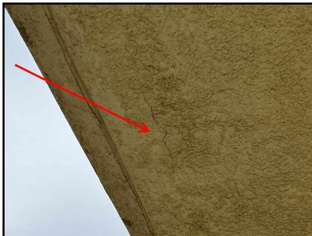
Photograph 3. Balcony edge spall.
