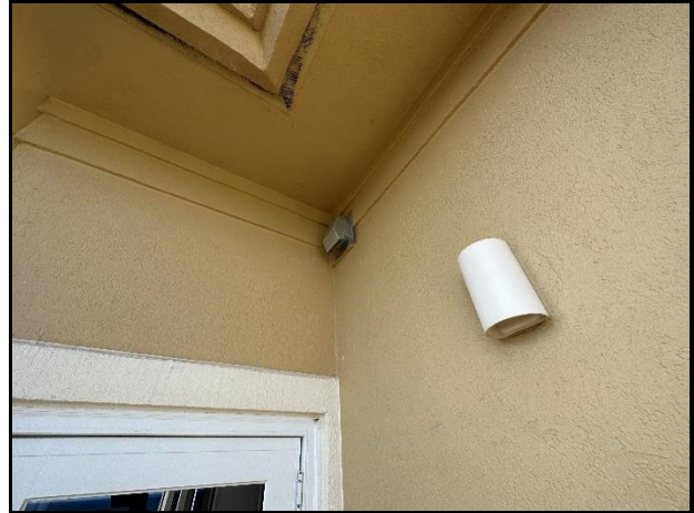
Photograph 18. Vent cover corroding.
