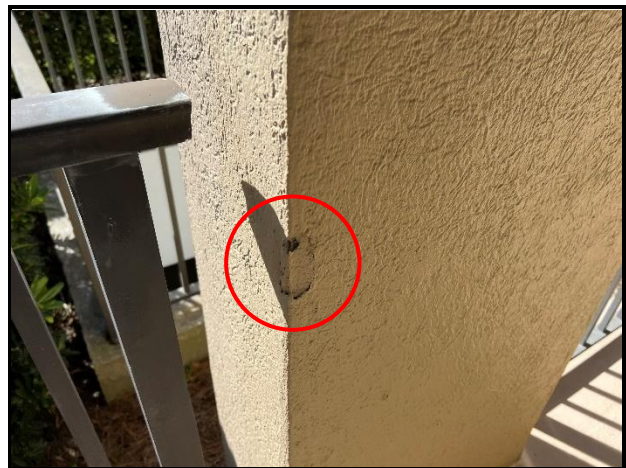
Photograph 16. EIFS impact damage.
