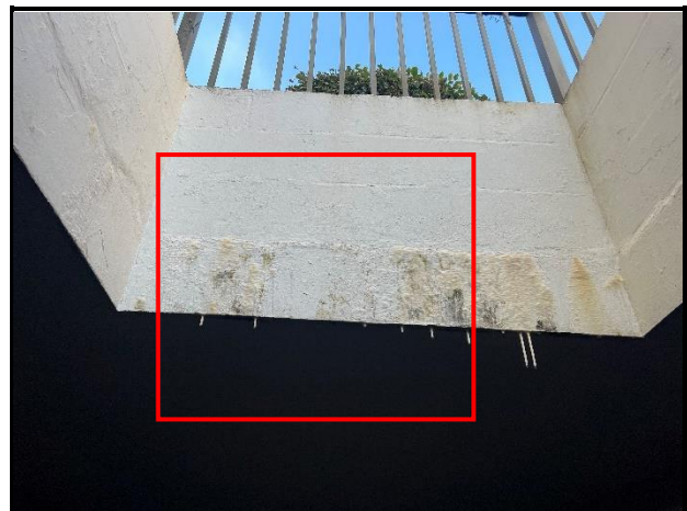
Photograph 28. Skylight with evidence of water intrusion.
