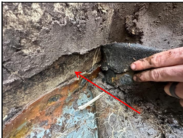
Photograph 27. Termination/perimeter sealant failed.
