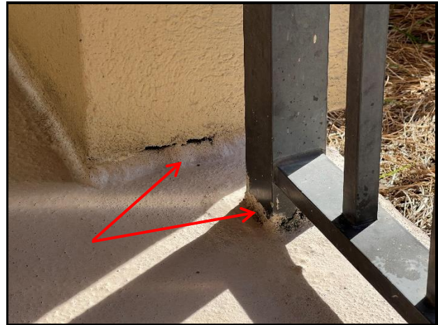
Photograph 12. Failed perimeter sealant.
