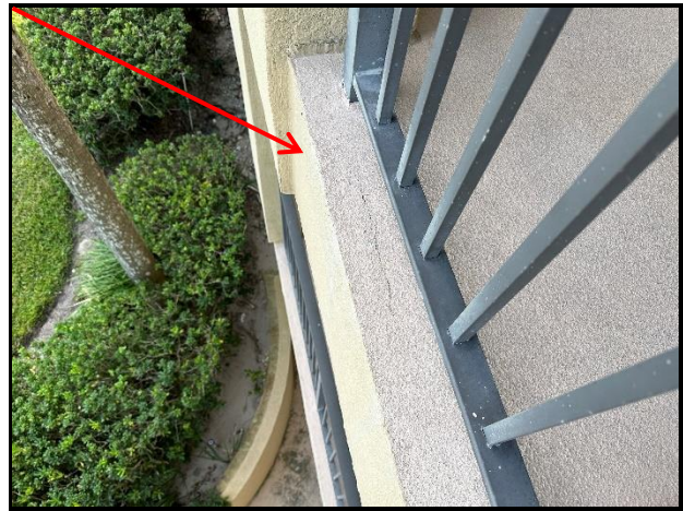
Photograph 2. Balcony edge spall near core mount.
