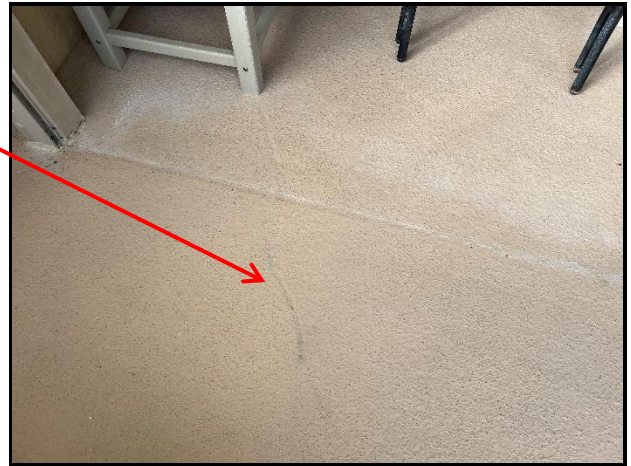
Photograph 6. Suspected crack developing in waterproofing.
