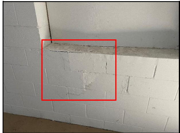
Photograph 24. CMU wall spall.
